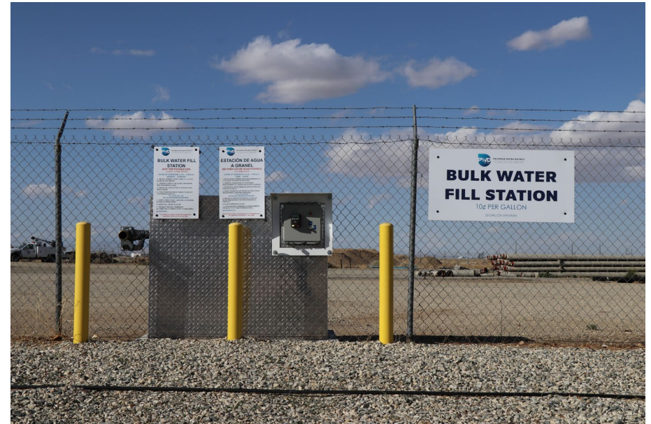
Photo of PWD non-potable fill station
